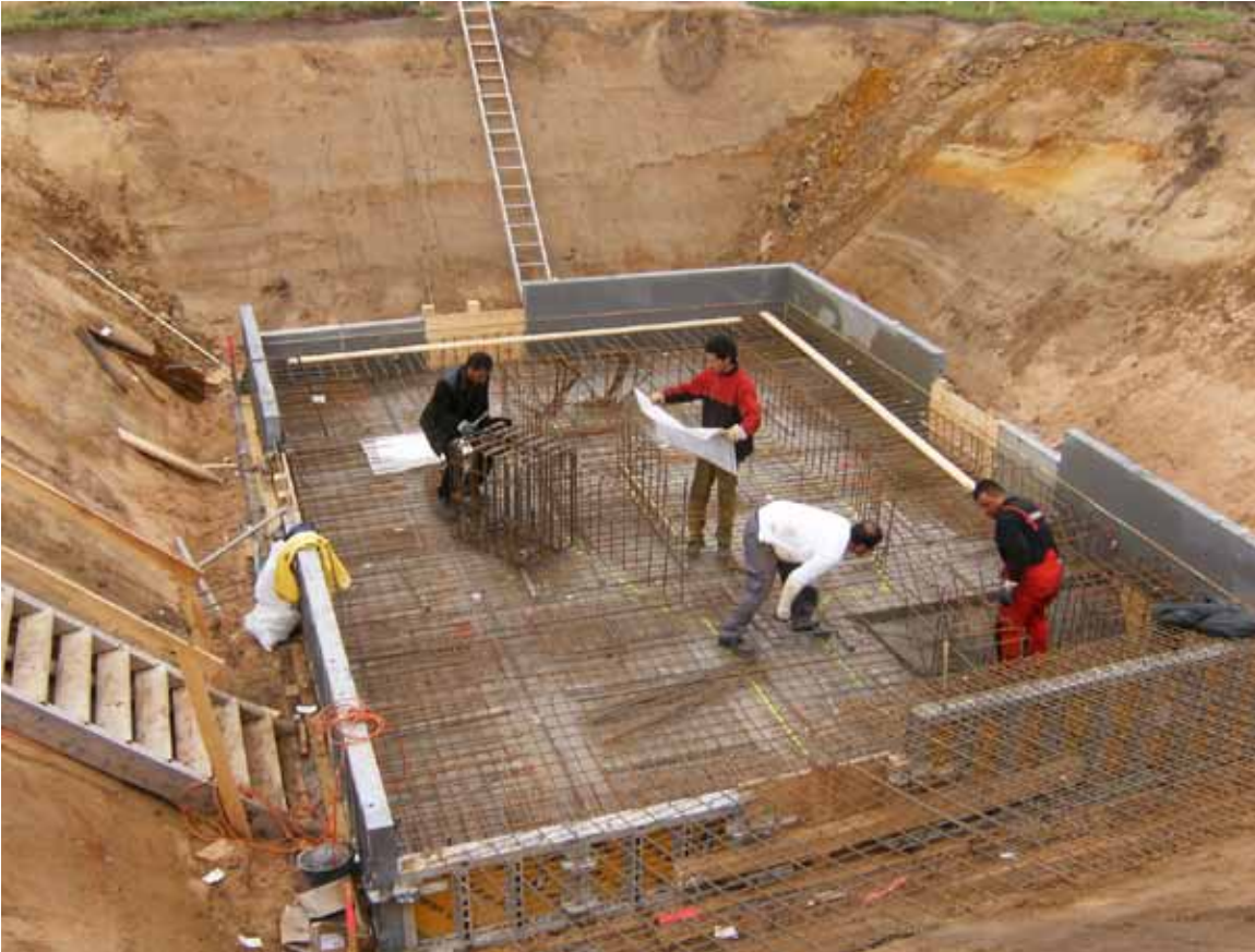
Engineers set the forms and rebar in the Universal Pit Foundation during a recent installation project.
